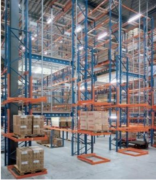
Fig. 16 VNA truck racking also supporting raised floors for order picking
